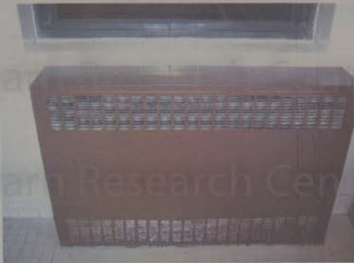
Students in the College of Nursing and Allied Health Sciences have had to endure harsh conditions due to malfunctioning heaters found in the building.
