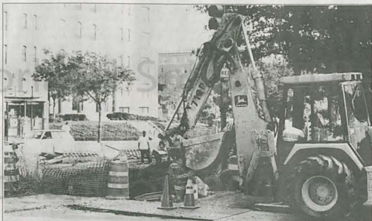
Photo by Chris Bell The construction in progress at the new Columbia Heights Metro station is making transportation difficult now.
