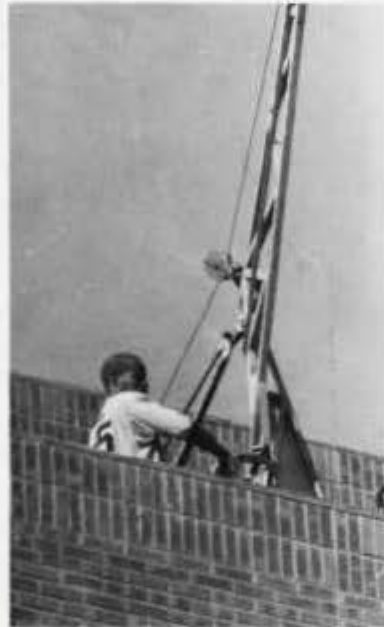
Worker lifts construction material to the roof of the new medical building. Photo by Keith Leadbetter
