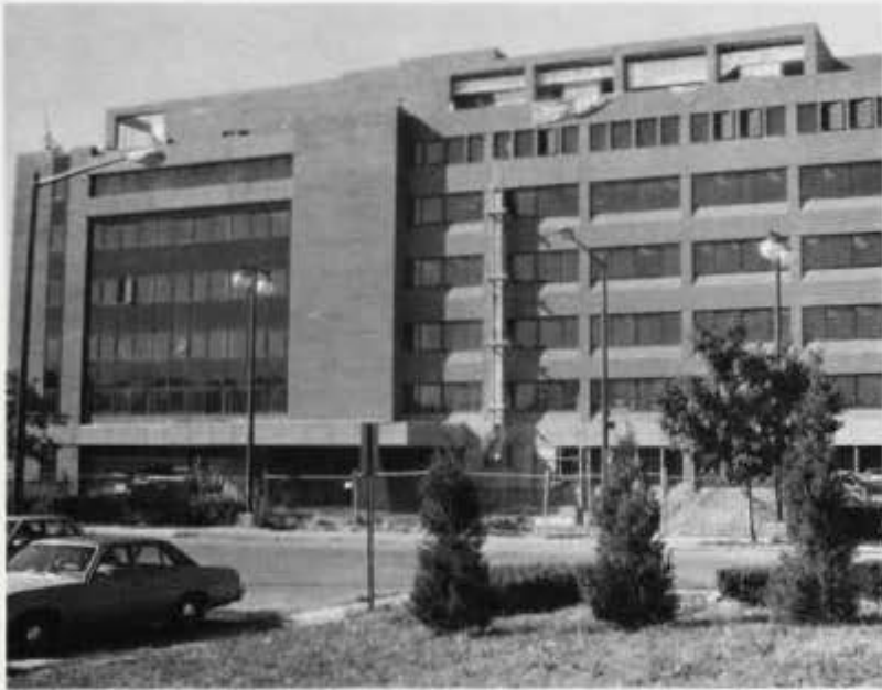
Construction continues on the Numa P.G. Adams Building. Photo by Keith Leadbetter
