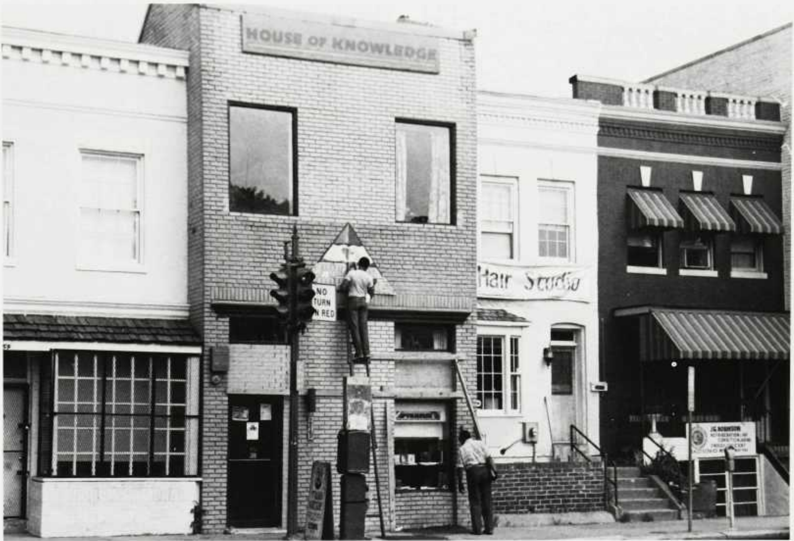
Building Pyramids. A worker helps to give the Pyramid Bookstore a new look.
