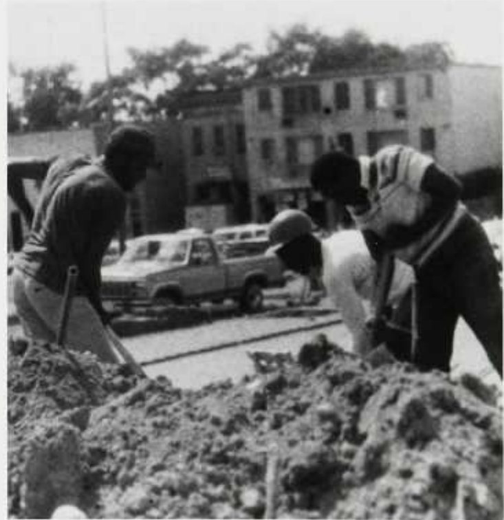
DIGGING DEEP. Before anything can be built, uneven land must be cleared.
