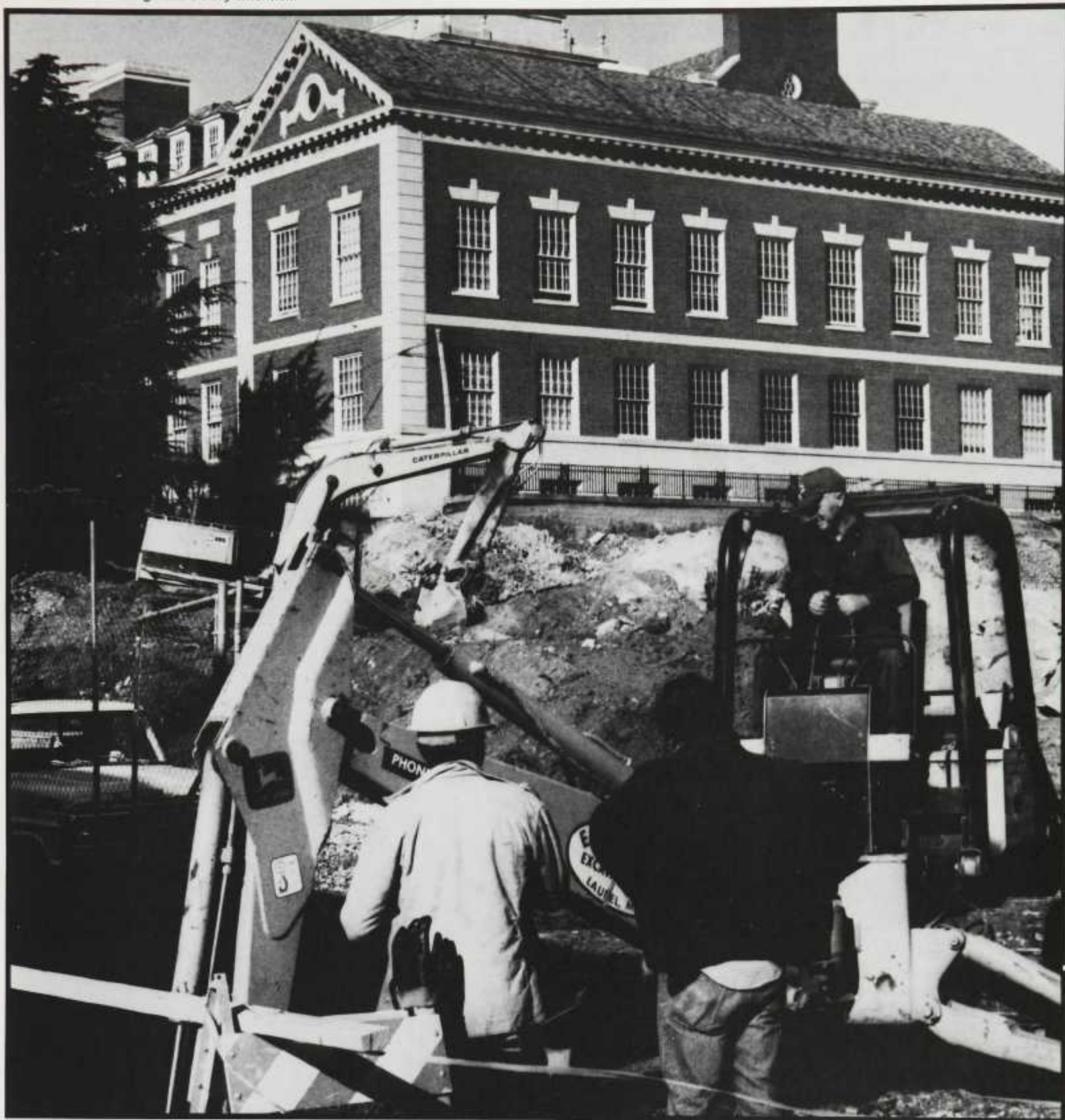
Clearing away the debris and dirt to begin construction on Founders' underground 3-story extension.
