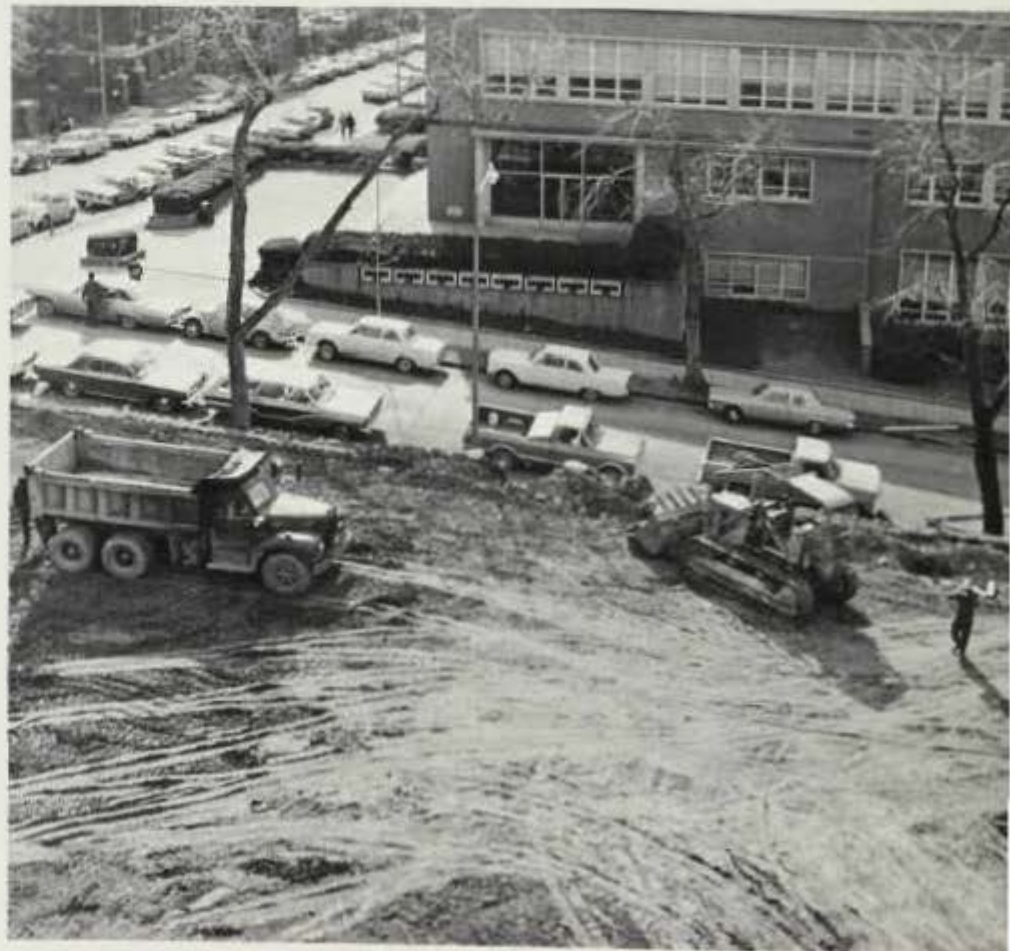
Ground breaking for the new School of Social Work began in February, 1969, and is to take several months to complete. Once the new building is completed, the old building can be torn down for the construction of the new Student Center.
